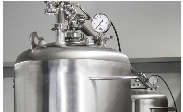
EL for pressure control installed in a tank
