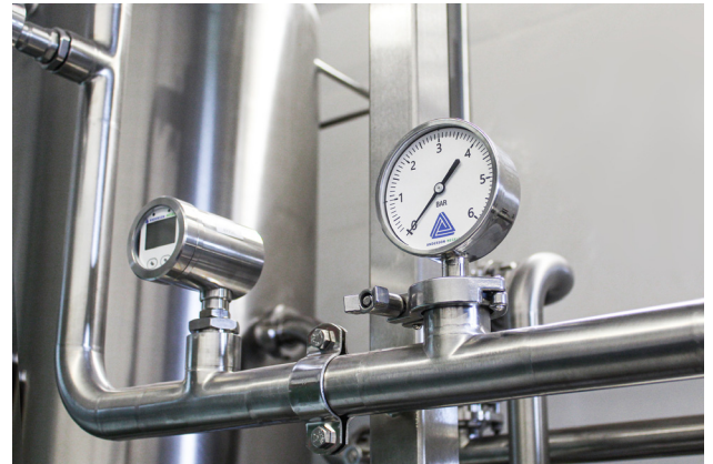
EL for process control installed in a pipe
