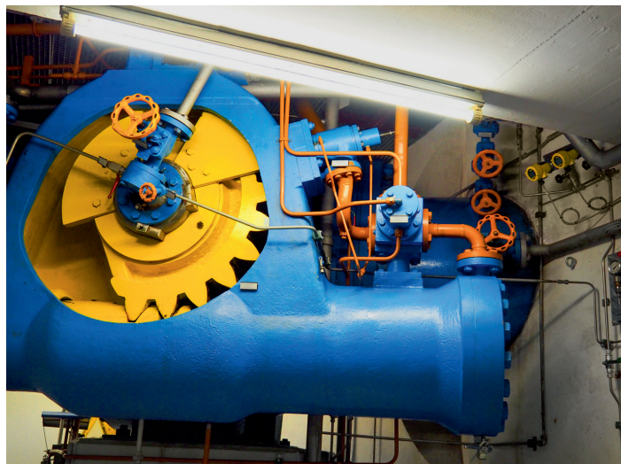
There are numerous sensors from VEGA not only in the dam itself, but also in the Roßhag power station. Compared to this huge shut-off valve, the two sensors are tiny.
